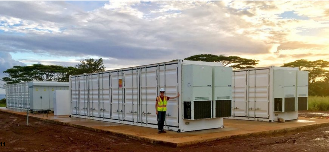
Representative image from earlier containerized BESS solution
